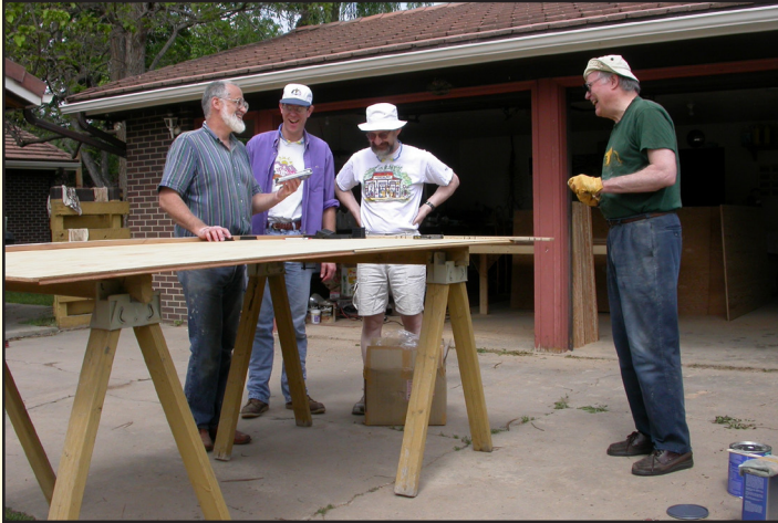
Phil Rice, Jerry Olson, Rod Frehlich and Dan Anderson joined the volunteer crew building the new floor.
